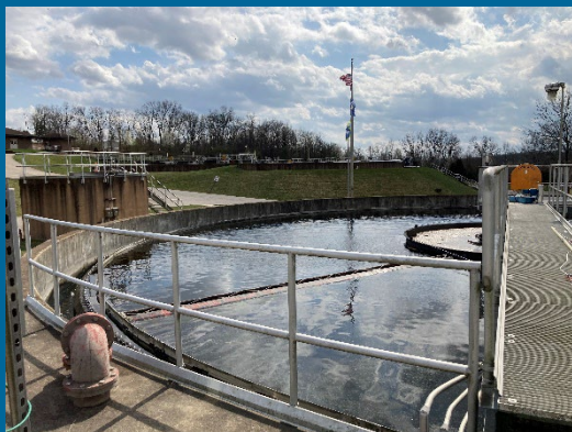
Floyds Fork Wastewater Treatment Plant
