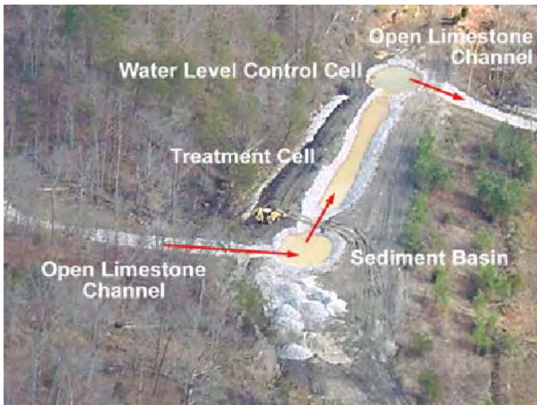
Figure 4. Paint Cliff Vertical Flow System Components (Phase I) (from Carew et. al., 2003)
