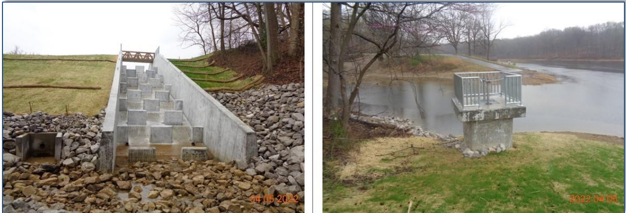
Scenic Lake Dam: new spillway and riprap stilling basin (L) and drawdown system tower (R)
