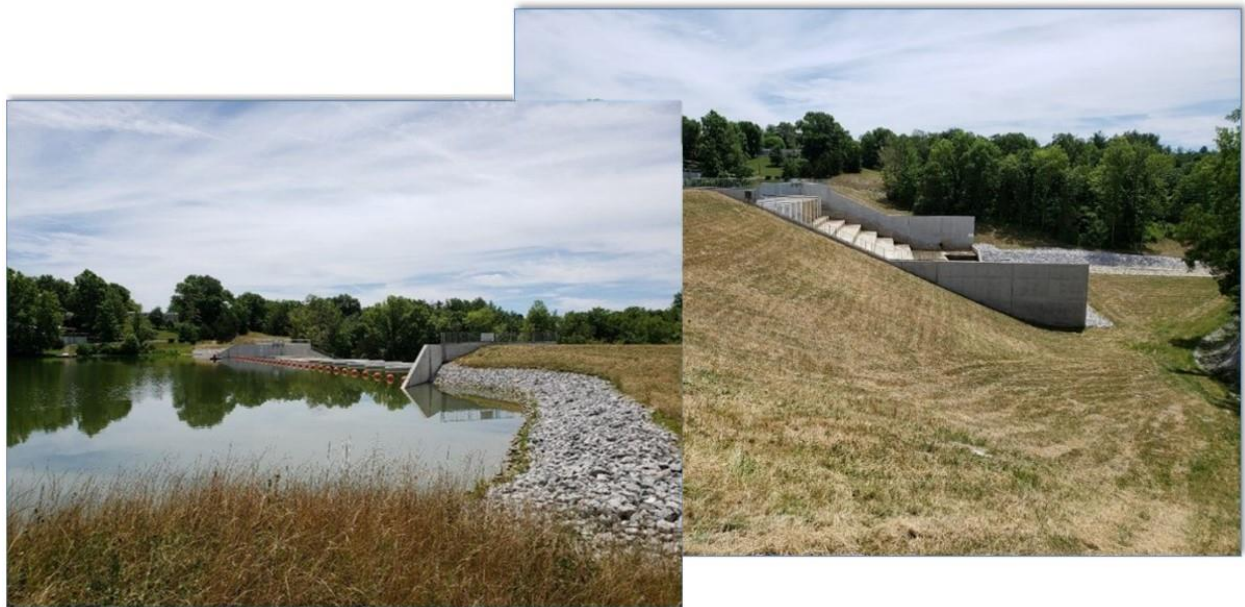
Bullock Pen Dam: right embankment and spillway view from lake (L) and from downstream (R)
