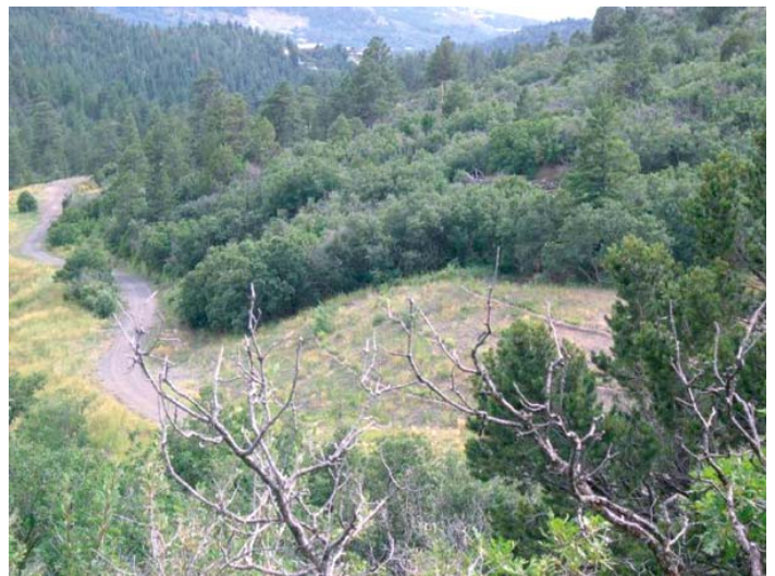
Franks Mine site following construction. (with relocated road and restored stream to extreme left of photo)
